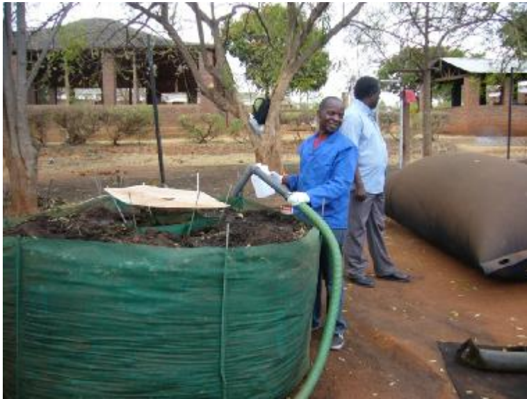
Flexigester 'Donut' for effluent disposal and gasholder full of biogas, June 2014
