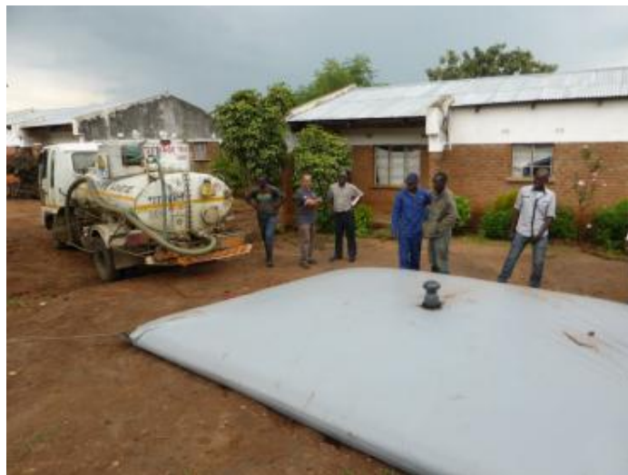
Emptying bladder/ Transfer station
